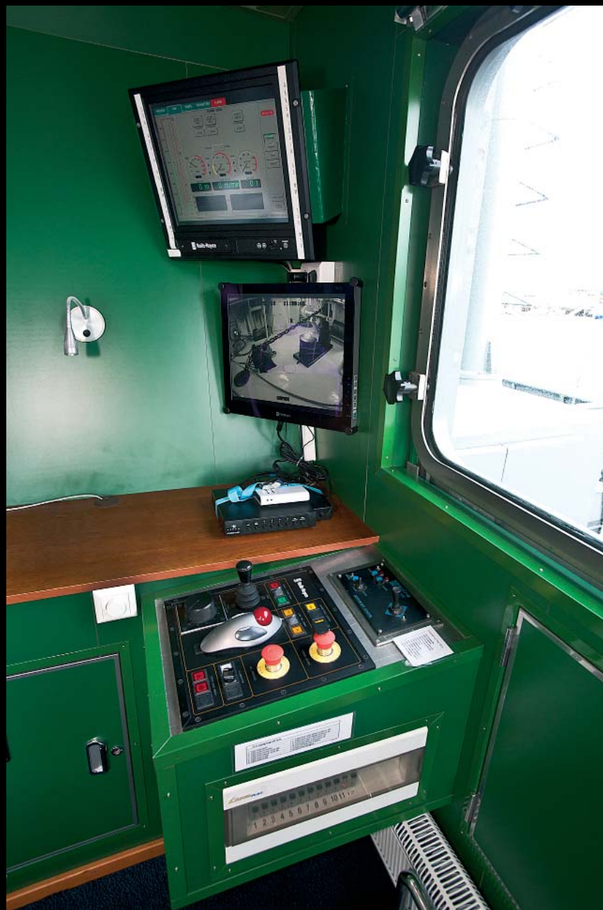
Salvage winch control and display and CCTV display
